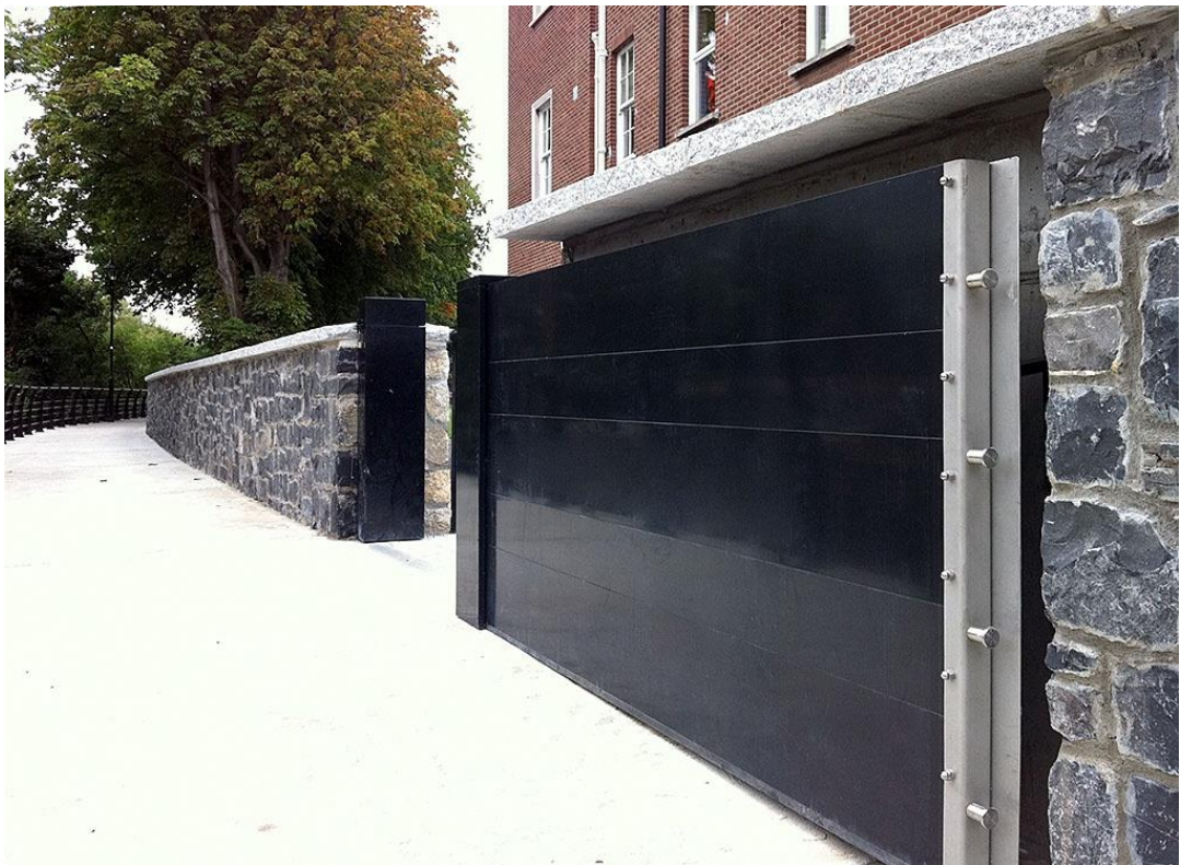
Fig. 24: Lift-hinged flood gate at Dodder Flood Protection Scheme
