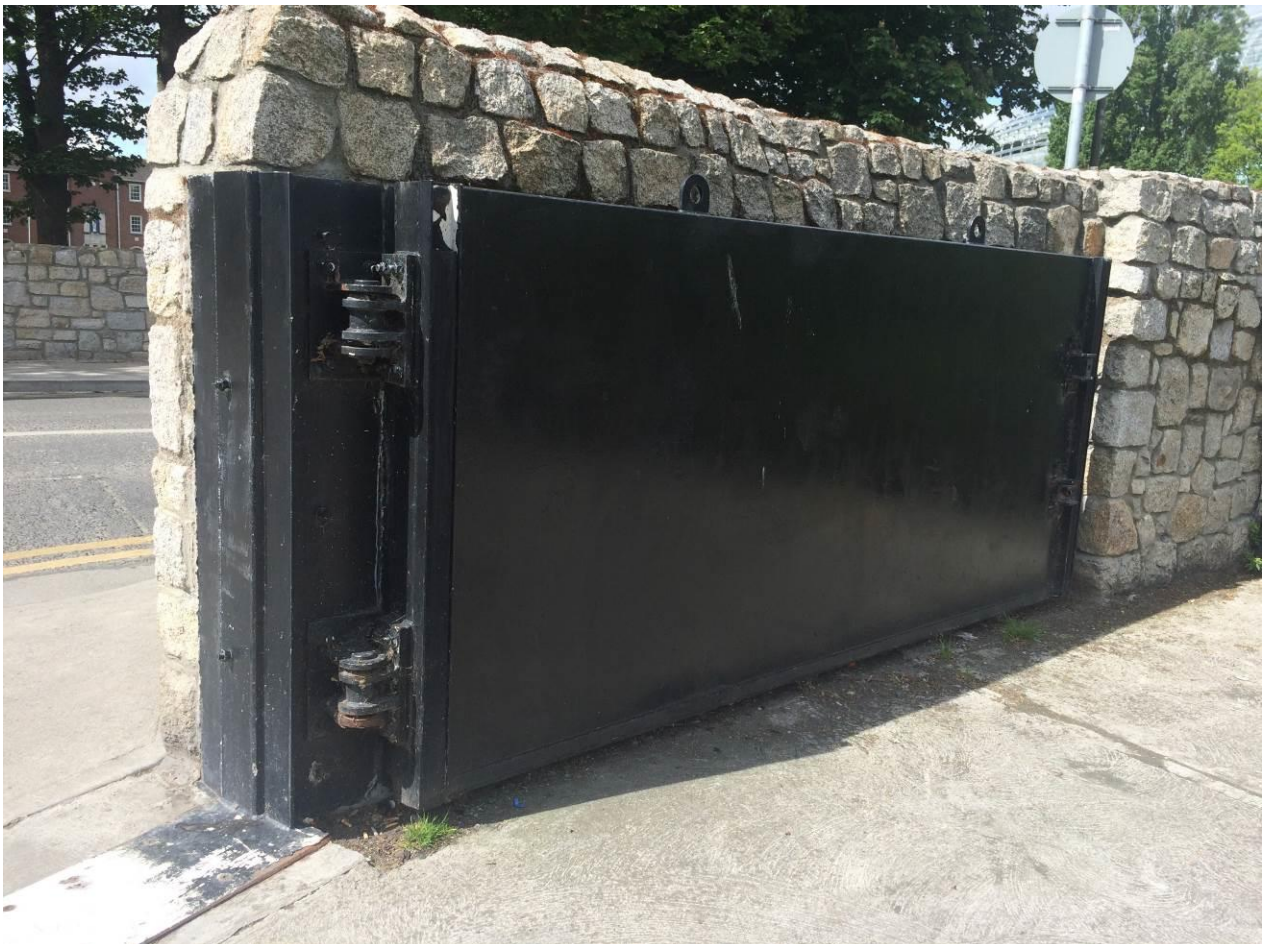
Fig. 27: Swing-hinged flood gate at Dodder Flood Protection Scheme
