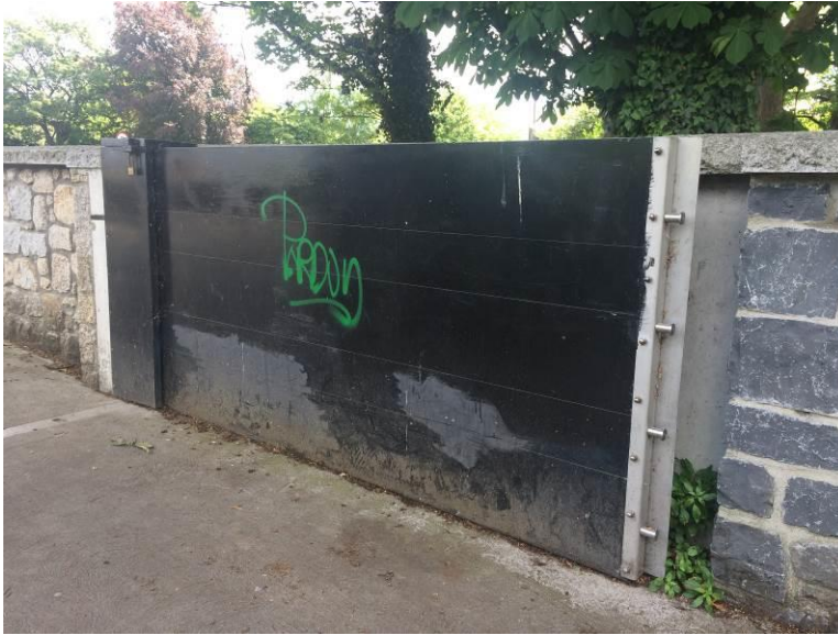
Fig. 25: Lift-hinged flood gate at Dodder Flood Protection Scheme
