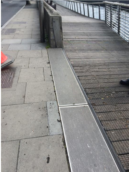
Fig. 30: Barrier in open position
