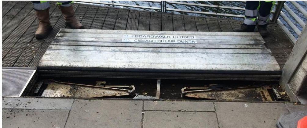
Fig. 28: Trench in which supporting fins and folding barrier are stored (Liffey Boardwalk)
